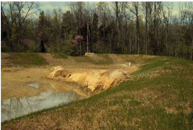
A leaking pond located in central Pennsylvania.
